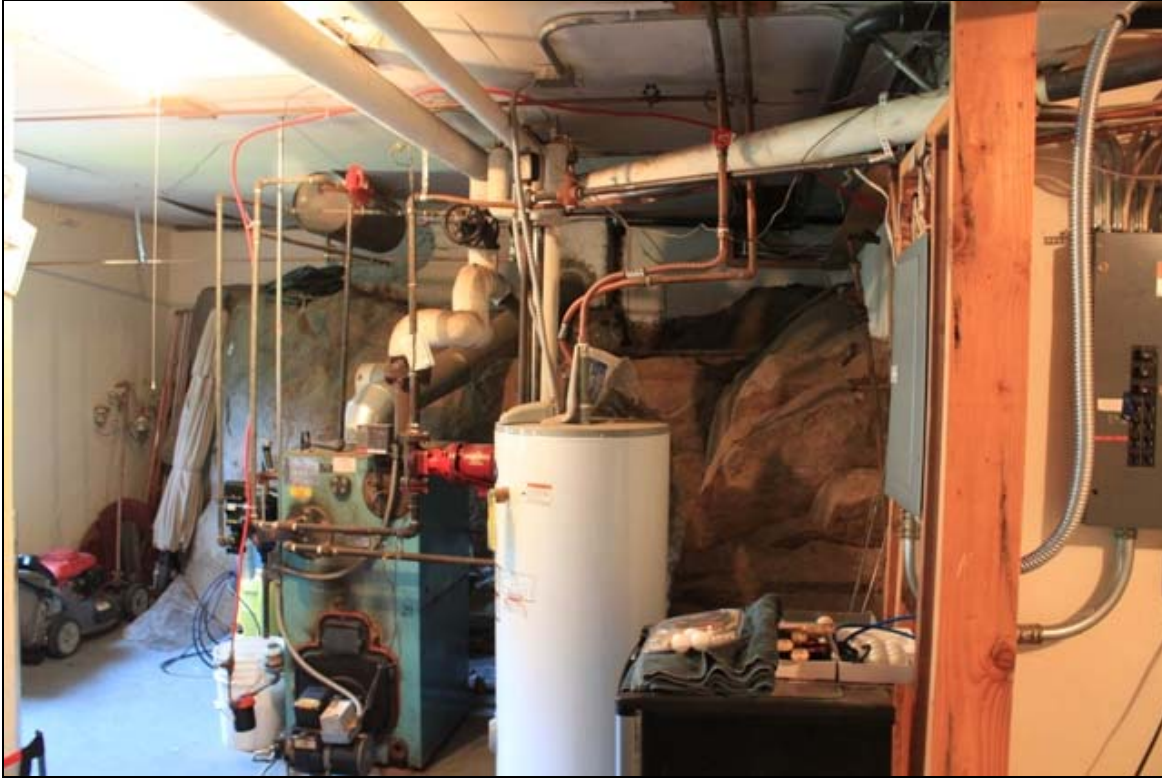
Photo 15 of 15: (OR_ClackamasCounty_OscoC.RoehrHouse_0015) Basement, steam heating system detail, camera facing west
