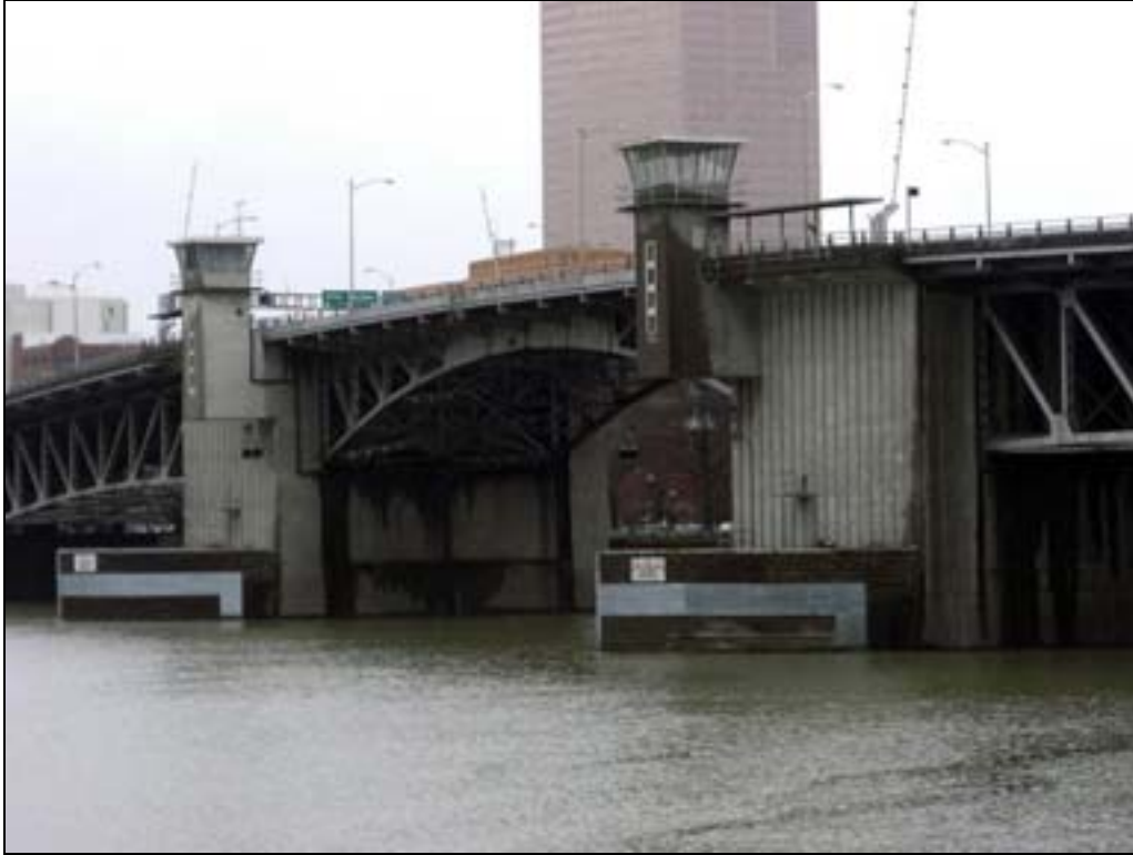
Photo 3 of 5: (OR_MultnomahCounty_WillametteHwyBridgesMPD_MorrisonBridge_0003) Bascule and Pier detail, looking NW, from Vera Katz Esplanade
