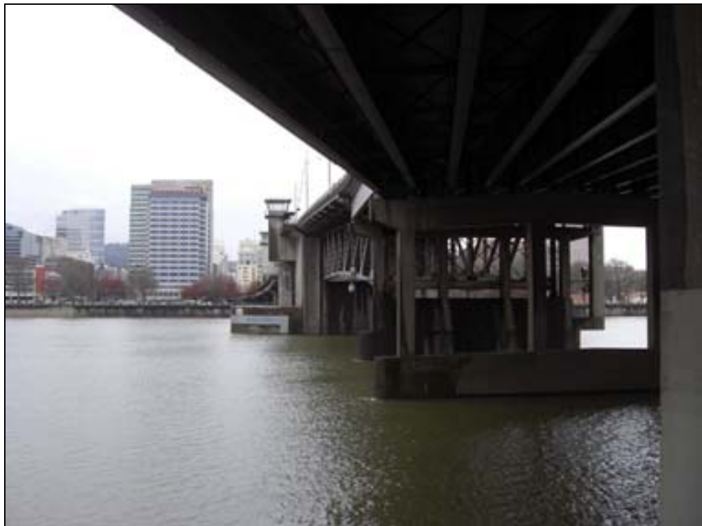
Photo 4 of 5: (OR_MultnomahCounty_WillametteHwyBridgesMPD_MorrisonBridge_0004) Understructure and "tower" view, looking West, from Vera Katz Esplanade
